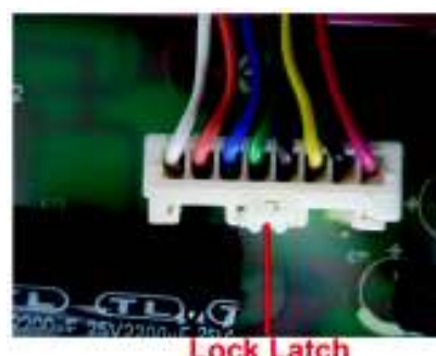
Cable Plug on DP
